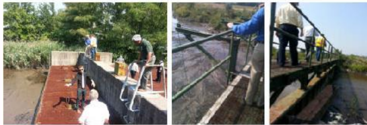
Figure 3-1: Physical Inspection of Existing Risk Reduction Infrastructure. Teams assigned by the New Jersey Department of Environmental Protection have endeavored to catalogue Superstorm Sandy’s impact on berms, tidal gates, and other existing risk-reduction infrastructure. Physical inspection is a key part of the State’s assessment of the current condition of measures to identify necessary repairs as well as opportunities to enhance existing measures to address future extreme weather events and maximize federal investment.
