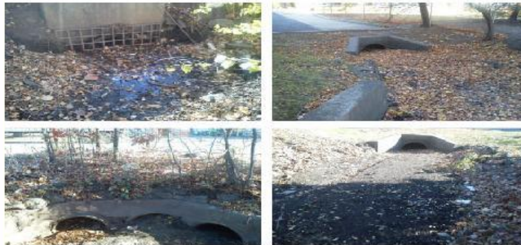
Figure 3-2: Drainage Systems, Moonachie/Little Ferry. Addressing drainage issues could offer low-cost investment opportunities to increase New Jersey’s flood resilience. For example, bottlenecks in drainage systems, accumulated debris, and overgrowth may collectively exacerbate the impact of flooding and storm surge on communities. In addition, some drainage systems, constructed piecemeal over the last two centuries, have never been mapped. For example, Rutgers has been evaluating how minor drainage improvements can reduce flooding in the Moonachie/Little Ferry region (pictured).
